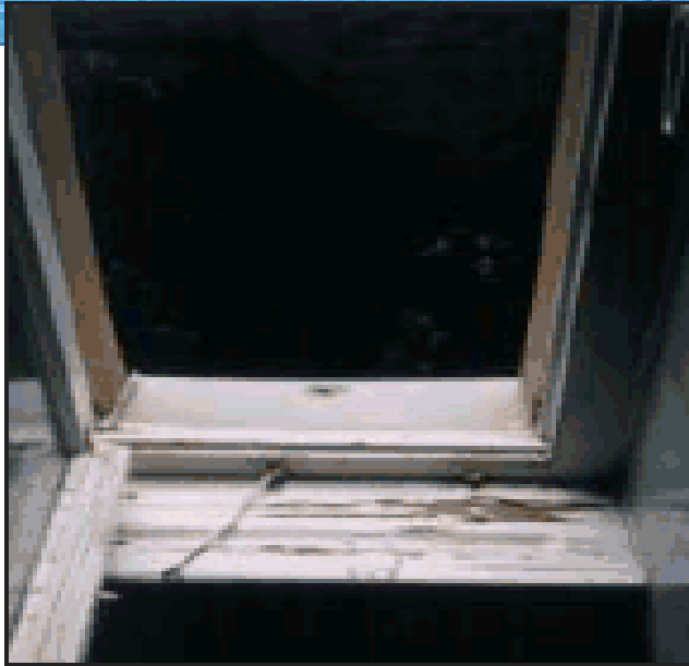
Leaky window – mold is beginning to rot the wooden frame and windowsill.
